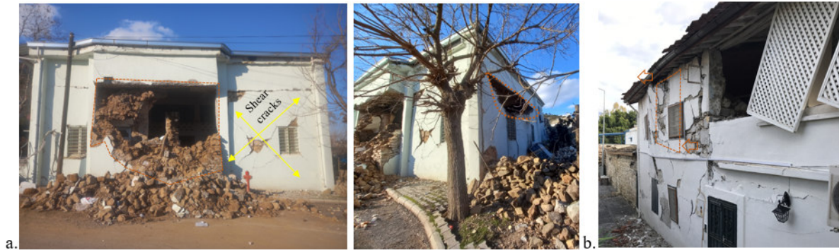
Figure 6. a. Out-of-plane failure wall collapses and in-plane shear cracks along with partial collapse of the transverse wall b. Bulging of masonry wall due to out-of-plane behaviour In another structure damaged by in-plane shear cracks initially became vulnerable to out-of-plane vibrations. Thus, bulging occurred with out-of-plane movement (Fig. 6b).
