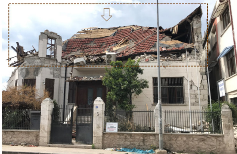
Fig.9. Upper floor collapse of a historic building in Antakya
