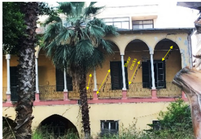
Figure 5. In-plane shear cracks in masonry walls
